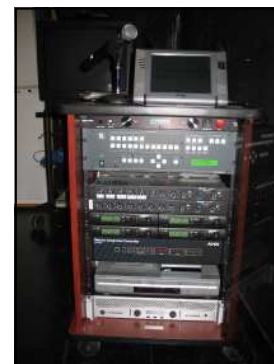
Main equipment rack
