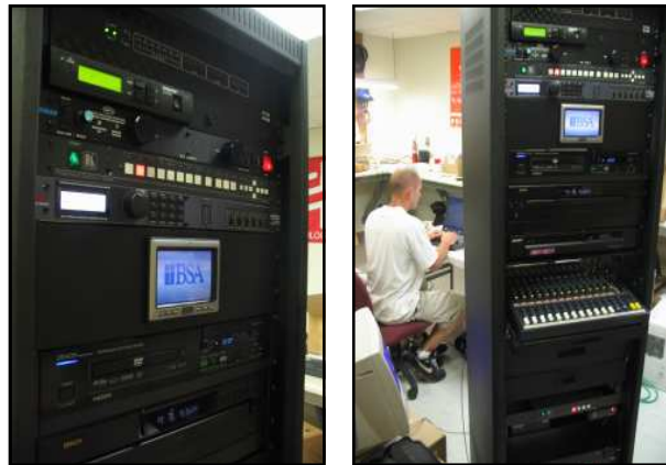
Main Equipment Rack
